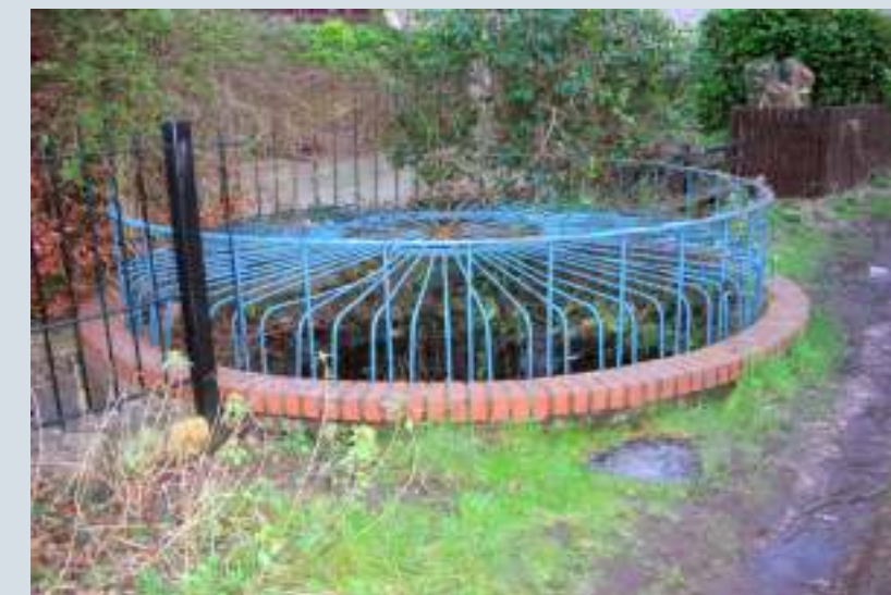
Bowbridge Circular Spill Weir
