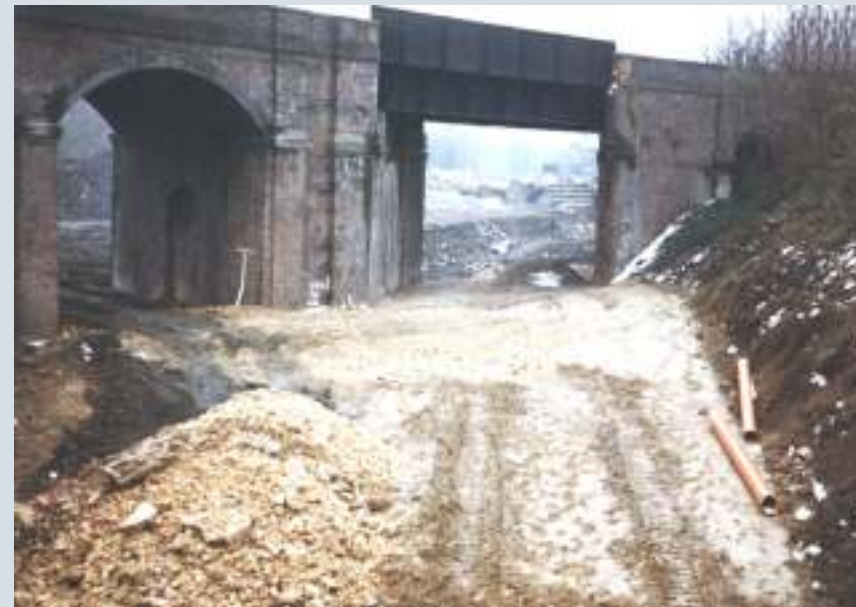
Capel Mill - construction of the by-pass on the line of the canal
