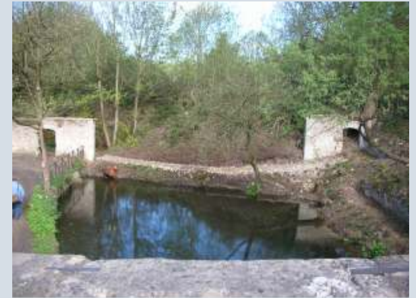
Contaminated Infill - at Brimscombe Port blocks the line of canal
